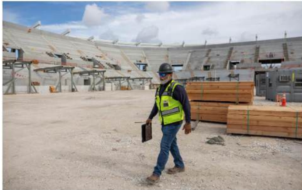
General superintendent on site for Lemartec, walks by as construction progresses at Miami Freedom Park stadium on Tuesday, June 24, 2025, in Miami, Fla. Photo by Matias J. Ochner mocner@miamiherald.com
